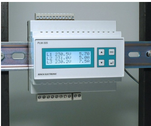
Power measuring device for energy analysis
